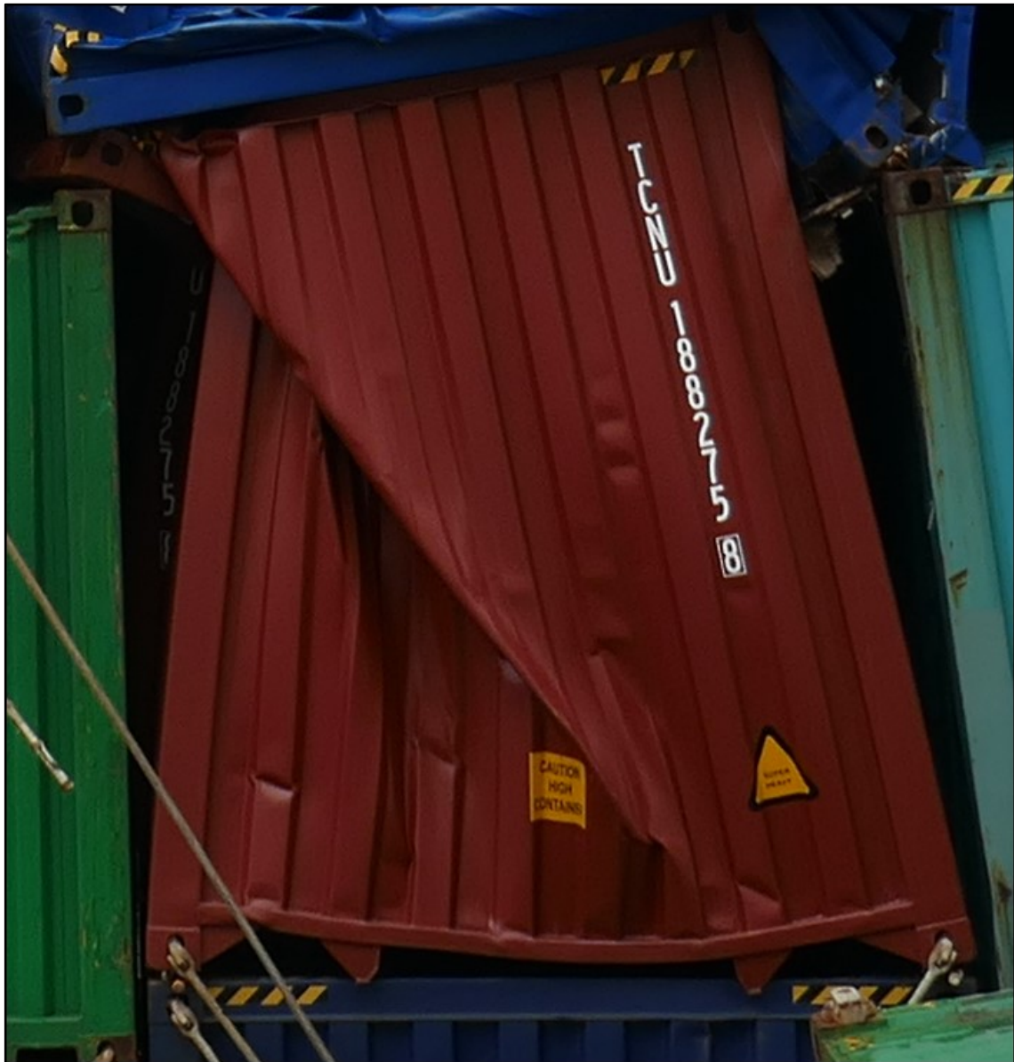
Figure 21: Image showing container corner post collapse
