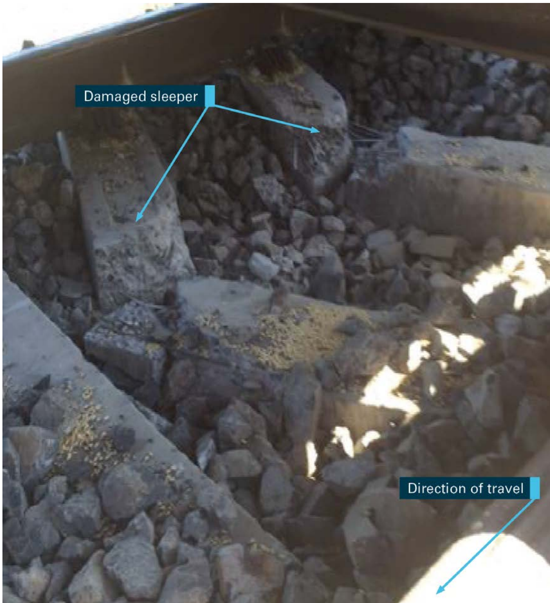
Figure 9B: Other damaged concrete sleepers
