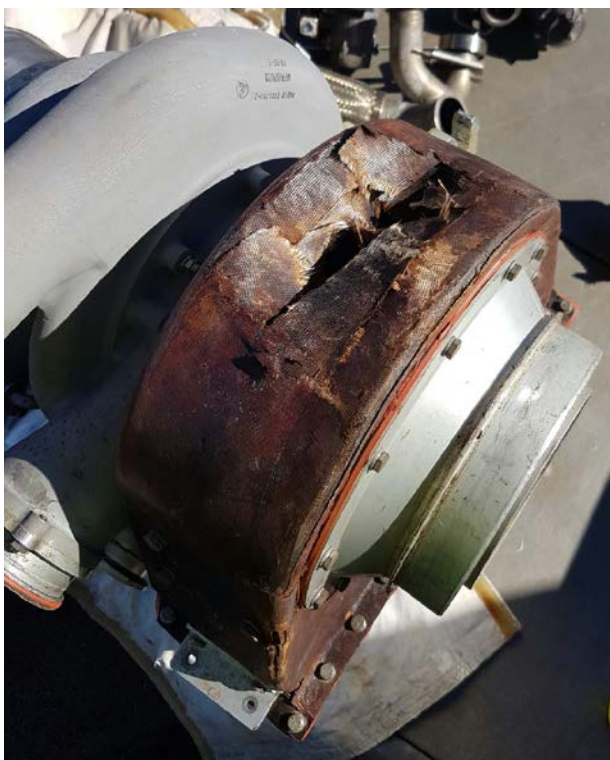
Figure 3: Ruptured plenum duct
