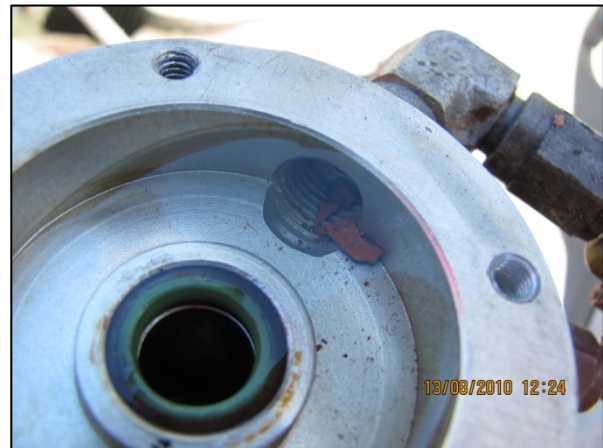
Figure 2: Fuel manifold valve with debris
