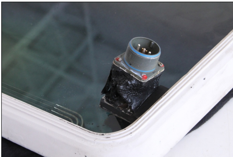
Figure 4: Close-up view of the melted terminal block
