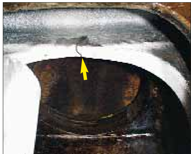
FIGURE 8: Crack (enhanced) through stiffening web in entablature at no. 4 unit
