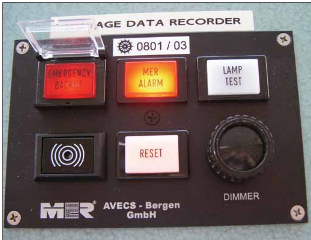
FIGURE 6: VDR wheelhouse control panel
