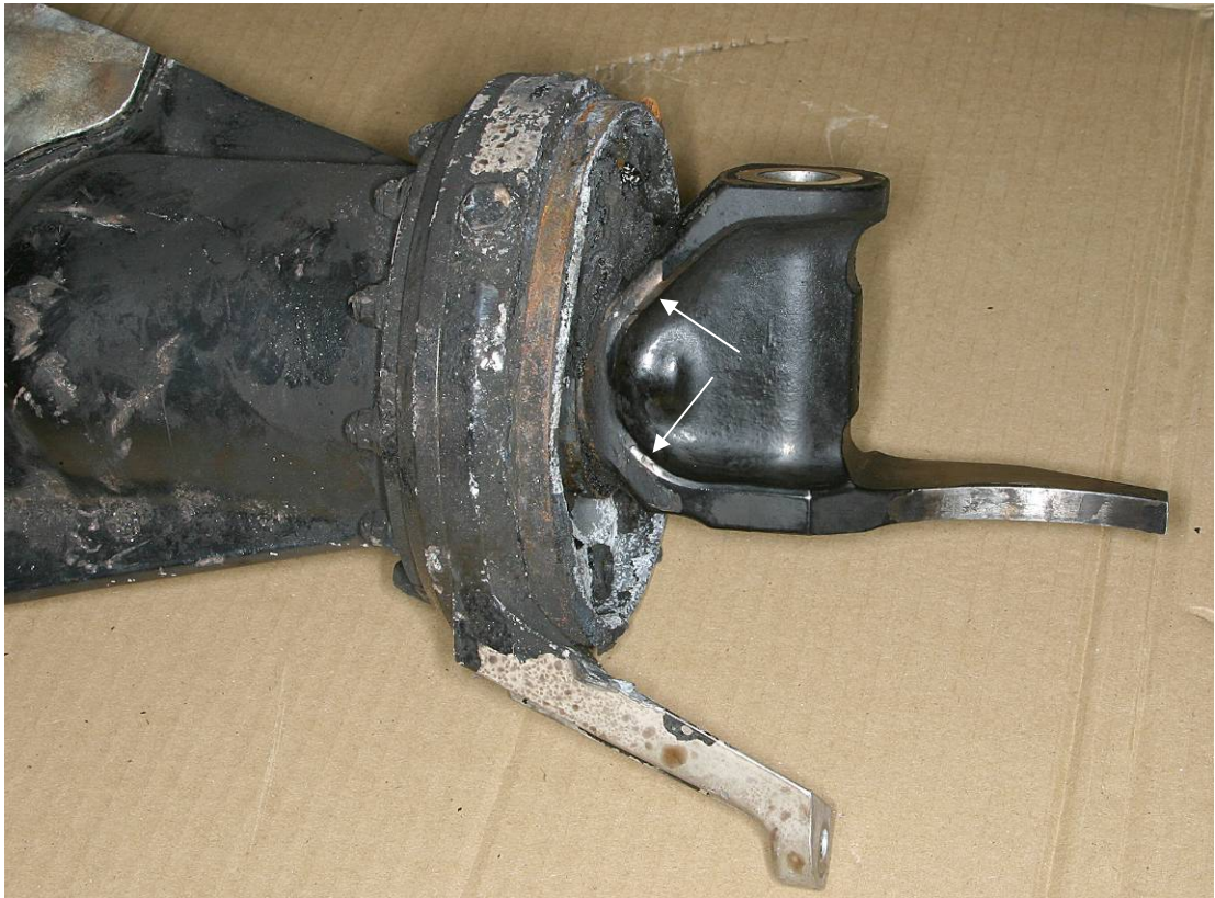
Figure 1: Hub assembly of blade S/N 4186-A showing general sound condition and absence of gross mechanical damage. Contact against the up-coning stops was evident (arrowed).
