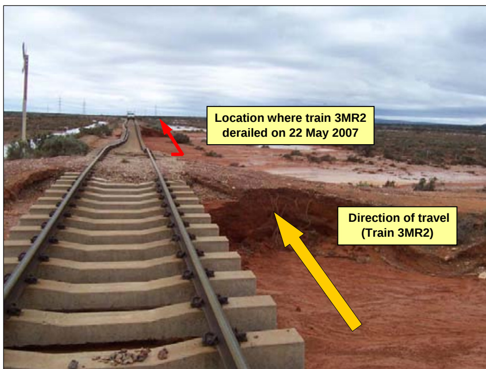
Figure 3: Track damage due to flooding (photograph, 22 January 2007)
