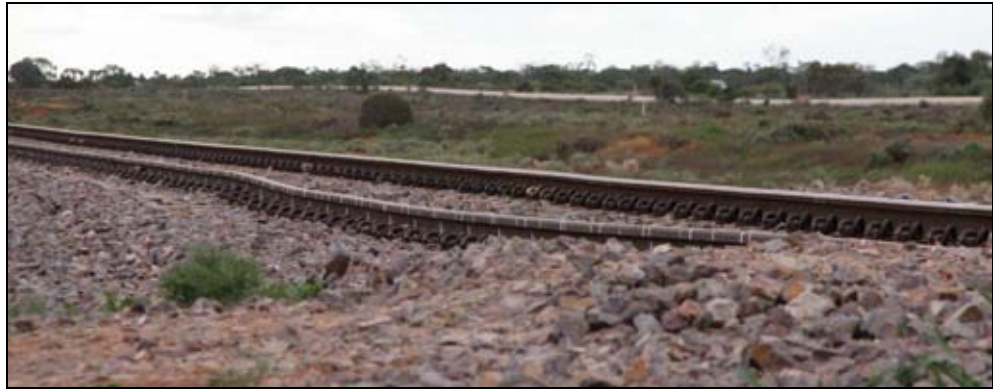
Figure 6: Track geometry defect (Photograph, 22 May 2007)
