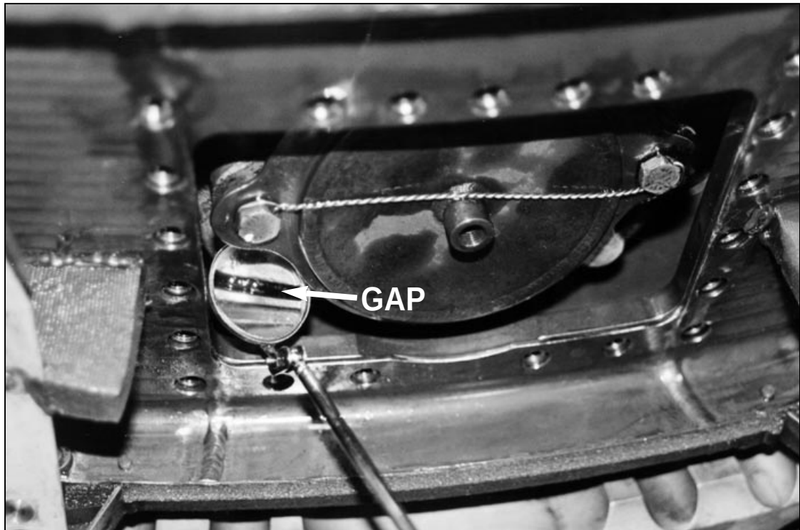
Figure 7. Partially detached angle gearbox housing cover.
