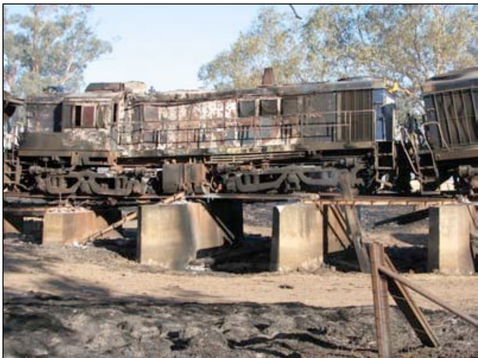
Figure 6: View of burnt out locomotives and bridge, note timber bearers of the bridge burnt from beneath locomotives
