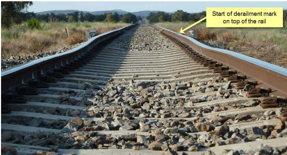
Figure 10: Track dip at the 538.588 km mark looking in the direction of travel
