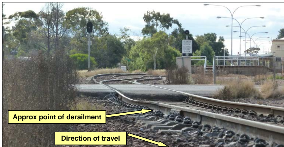
Figure 4: Track within the temporary speed restriction near the Carlton Parade level crossing.
