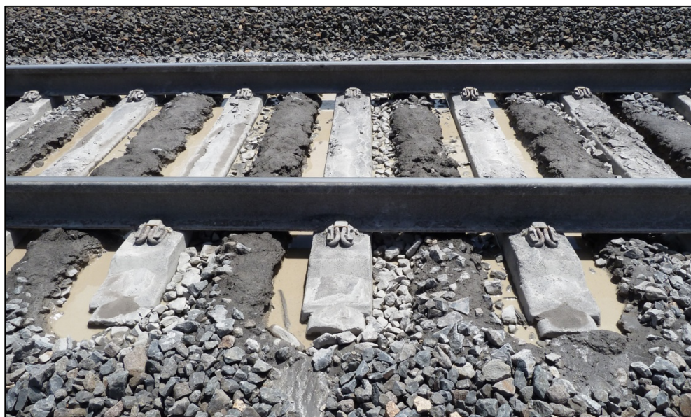
Figure 2: Typical mud-hole due to fouled ballast
