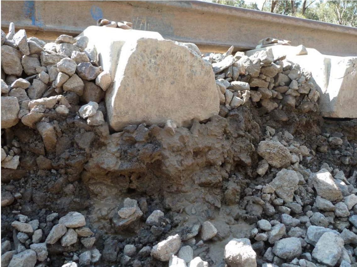
Figure 29: Highly fouled ballast under concrete sleepers
