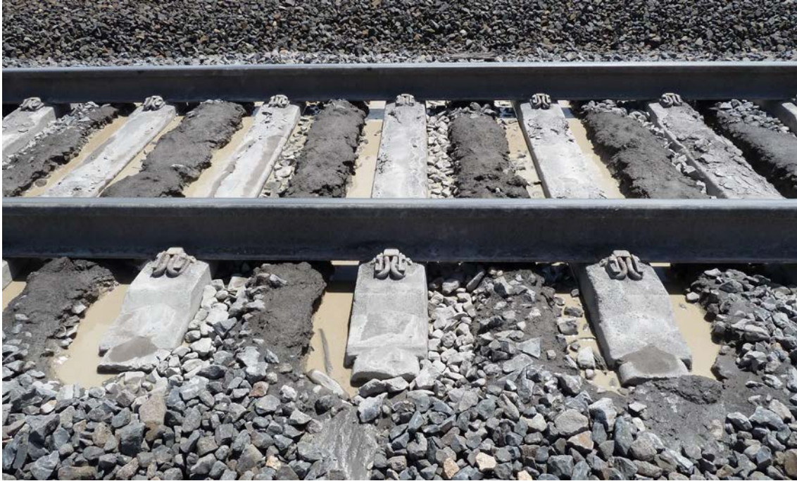
Figure 5: Typical mud-hole due to fouled ballast
