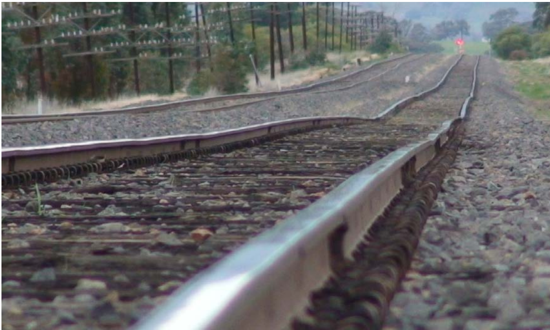
Figure 4: Poor track geometry
