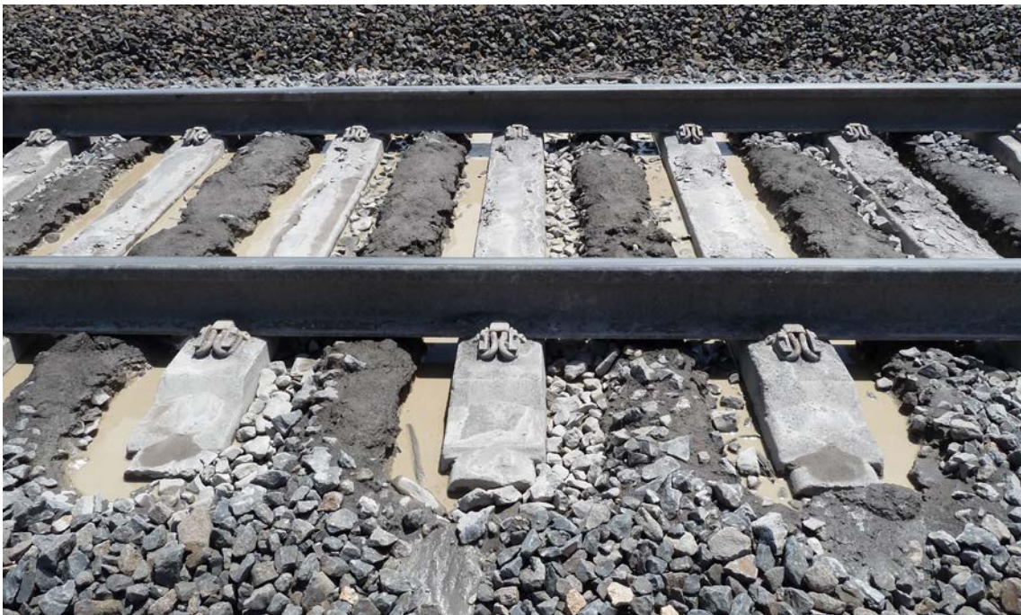
Figure 30: Water trapped within the track structure by highly fouled ballast
