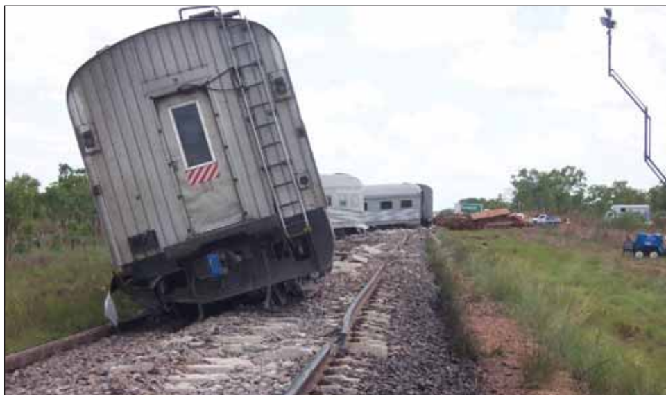
Figure 11: Damage to rail infrastructure in the vicinity of derailed carriages
