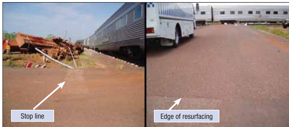
Figure 33: Left photo showing stop line barely discernible, right photo showing where road has been re-sealed with no barrier line
