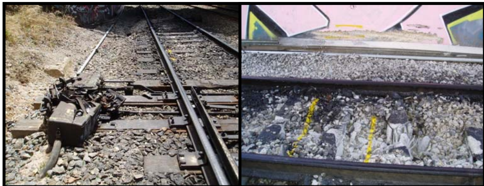
Figure 8: Damaged point machine (left), concrete sleepers, bridge abutment and cable ducting (right)
