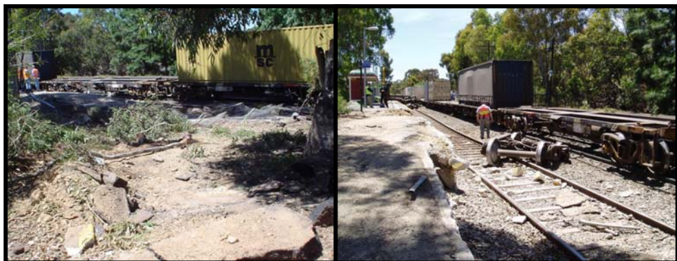
Figure 18: Damaged pedestrian crossing and passenger platform at Glenalta Railway Station
