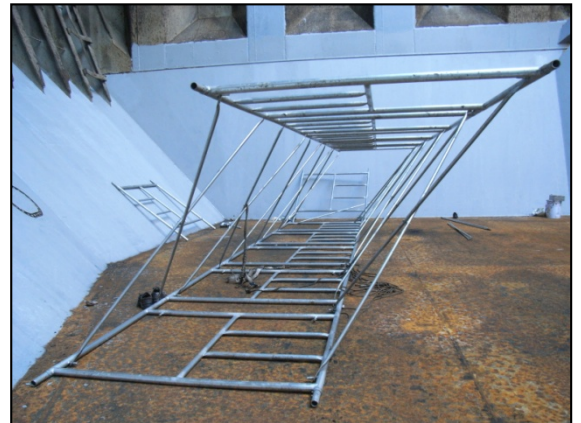
Figure 5: Twisted tower after the incident
