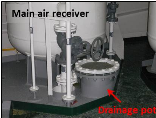
Figure 3: Air receiver condensate drainage pots
