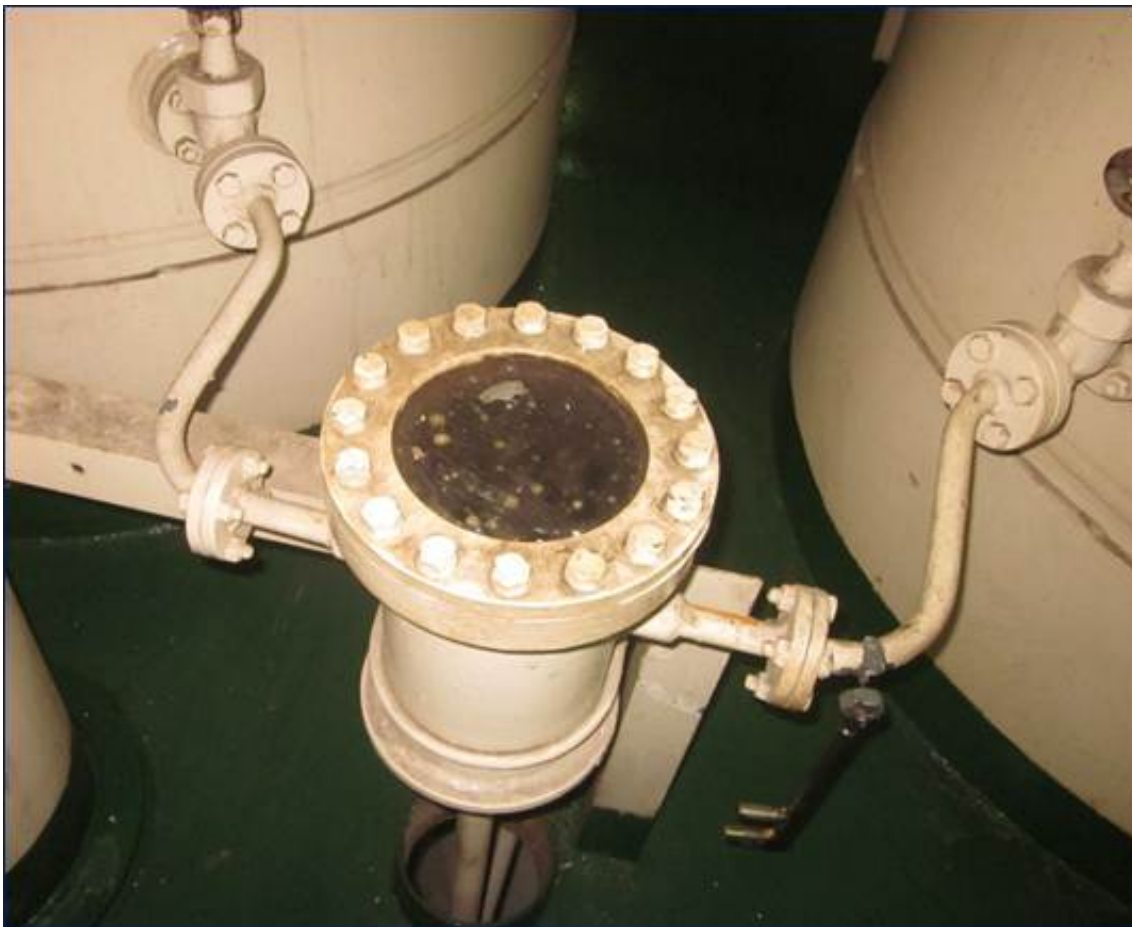
Figure 7: Similar design of condensate drain pot fitted on board another ship
