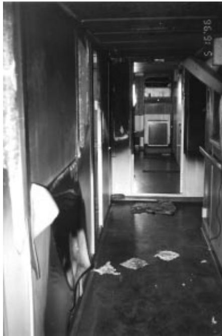
Heat and smoke damage in alleyway outside 2nd Engineer's cabin
