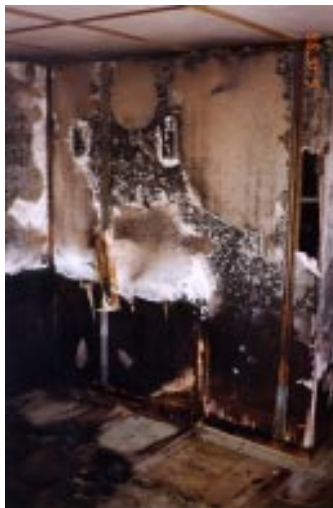
Fire damage to cabin windows and bulkheads
