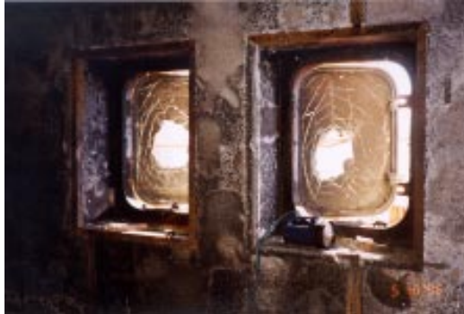
Burned area of vinyl deck tiles adjacent to 2nd Engineers bunk
