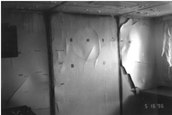
View from 1st Engineer's cabin of bulkhead between 2nd and 1st Engineers' cabins showing effect of heat transfer
