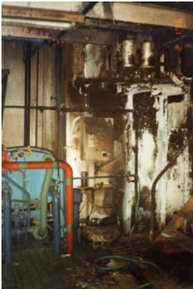
Starboard aft corner of seismic machinery space after the fire.
