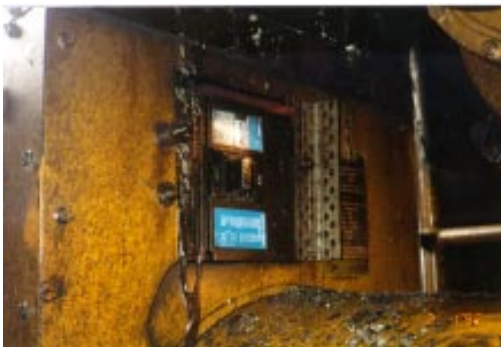
Circuit breaker fitted to seismic generator.
