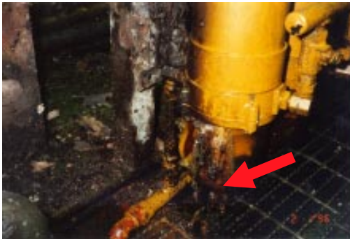
Melted polycarbonate fuel filter bowl on standard D399 compressor engine.
