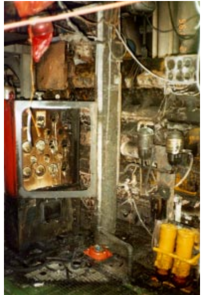
Fire damage to starboard D399 Caterpillar engine and control panel.
