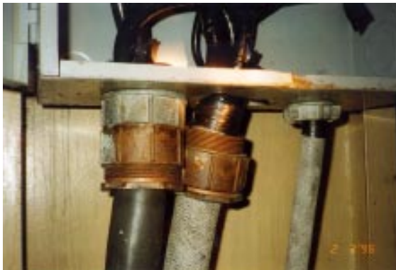
Aft end of same cable at seismic supply changeover switch showing poor standard of installation.
