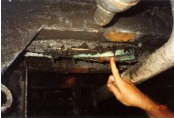
Damage to cable caused by short circuit between phases.
