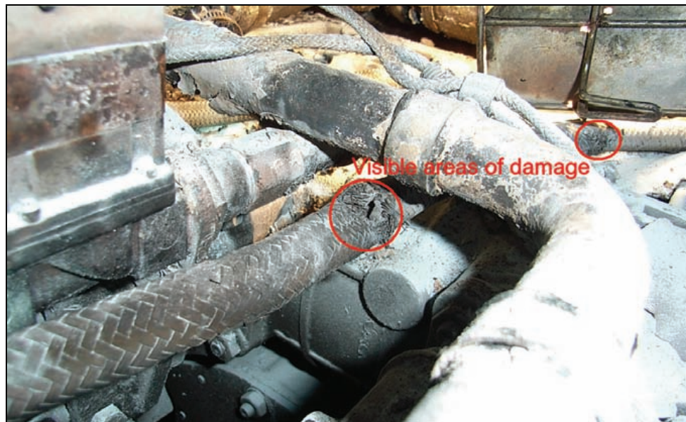
Figure 9: Failed 'filter hose' in situ with two visible areas of damage
