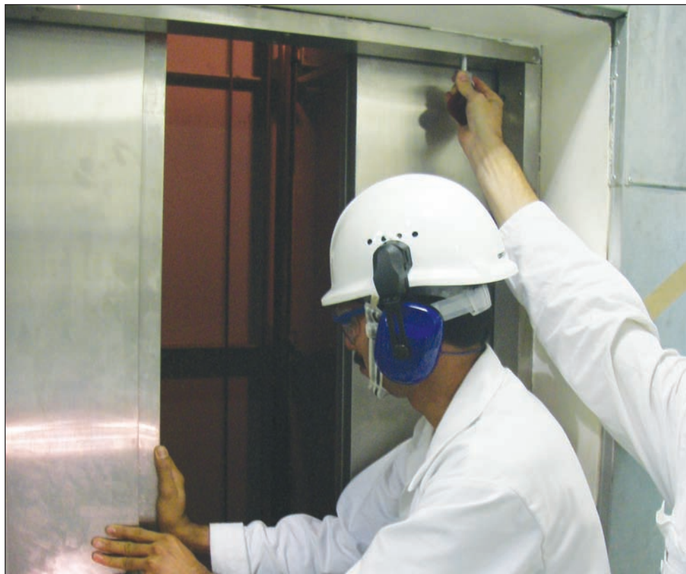
Figure 4: Elevator landing doors being manually opened
