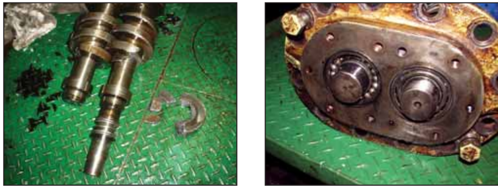
Figure 12: Broken pump scrolls and collapsed pump bearing
