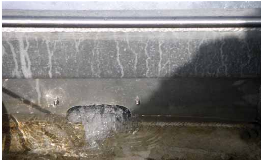
Figure 10: Water flooding the motor-well at slow speed
