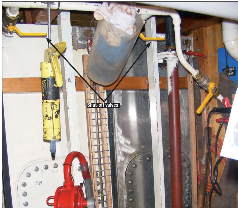
Figure 9: Shut off valves for air pipes
