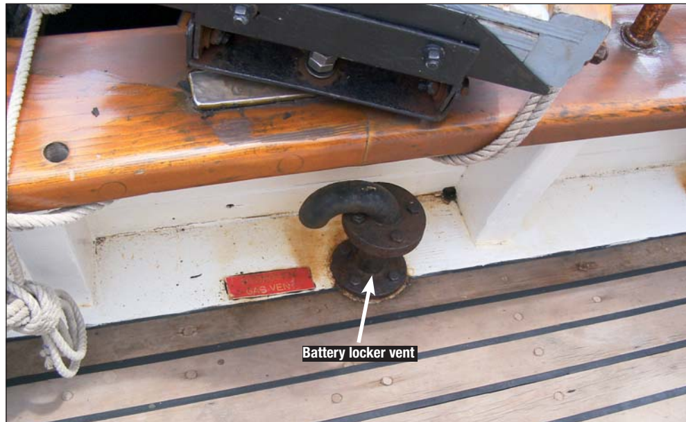
Figure 10: Battery locker vent
