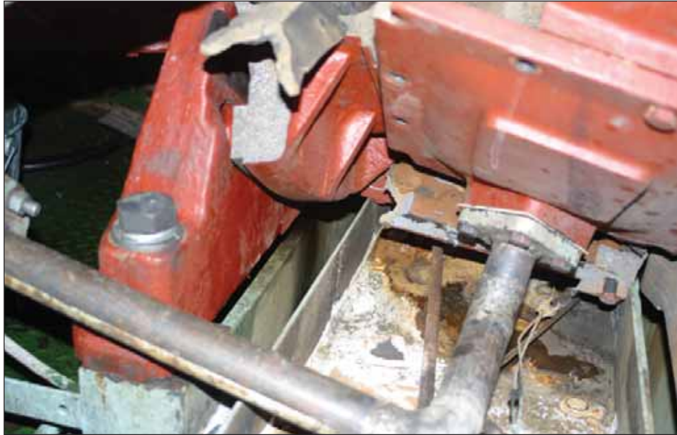
Figure 26: Failed housing mounts
