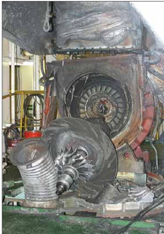
Figure 24: View of the second failed turbocharger showing the ejected shaft and exposed exhaust outlet casing
