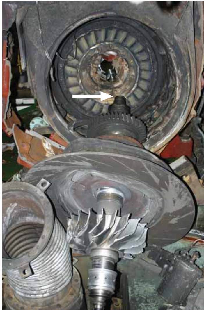
Figure 28: Shaft and turbine wheel ejected from the casing due to the failure of the shaft at the bearing housing (arrowed)
