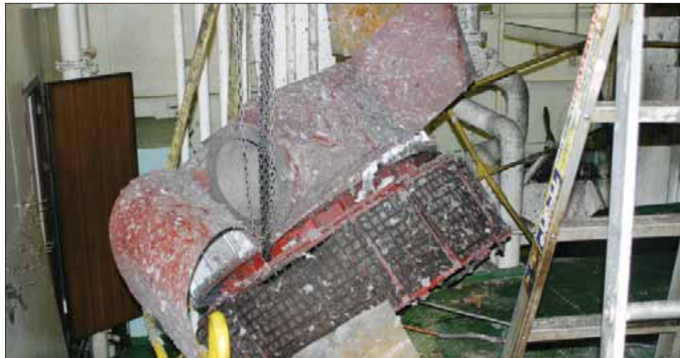
Figure 35 & 36: Compressor housing completely separated from the turbocharger body and exhibiting extensive internal damage
