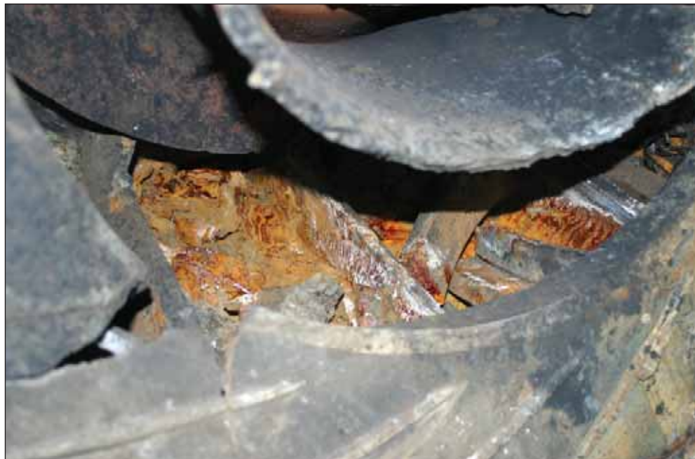
Figure 12: Debris and corrosion within the lower compressor housing body, indicating break-up of the cooling channels and the ingress of water
