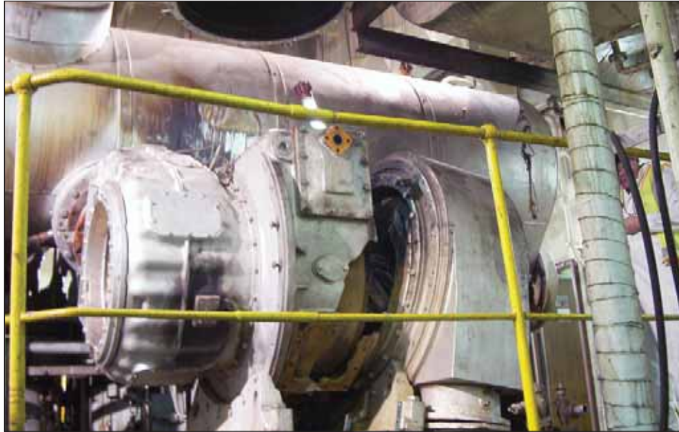
Figure 4: Failed turbocharger 22 September 2002
