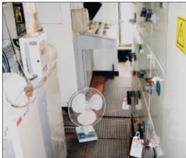
Inside number 1 cargo control room showing bucket elevator circuit breaker and the control panel
