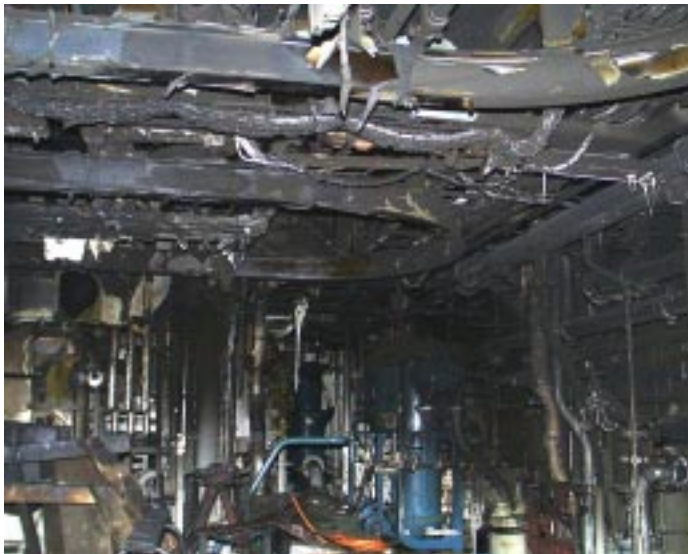
Damage to electrical cables under deckhead
