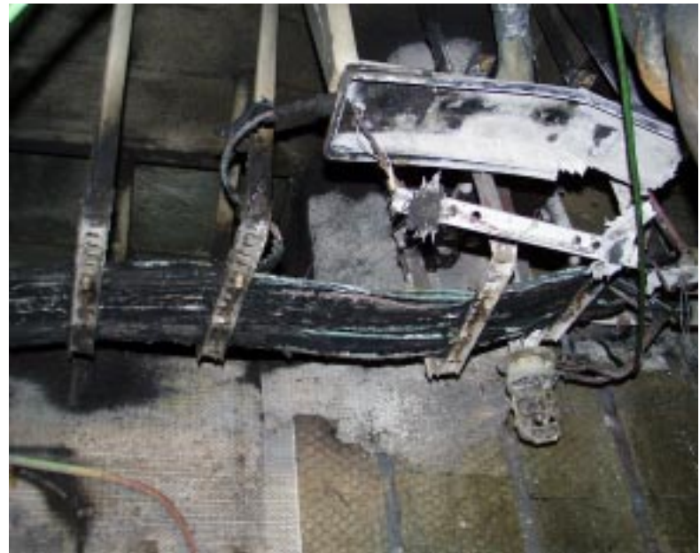
FIGURE 5 Fire damage to deckhead cables and fittings
