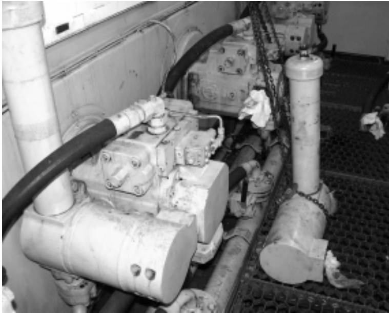
Hydraulic pumps (No.3 damper/filter unit removed)
