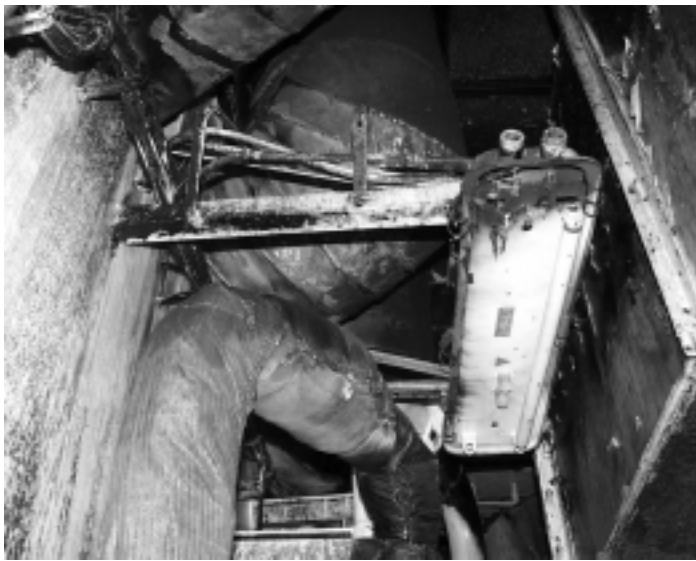
Fire damage immediately aft of hydraulic room bulkhead Small lagging fire occurred on this pipework
