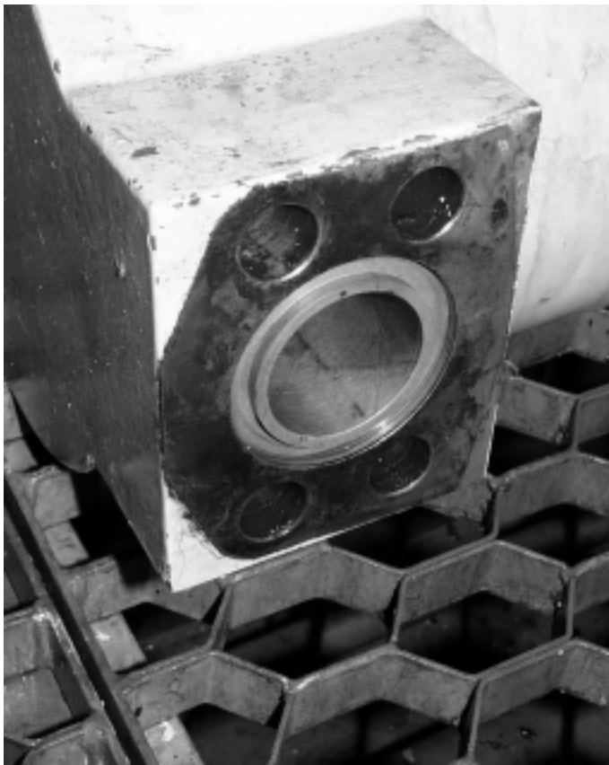
Damper body joint face
