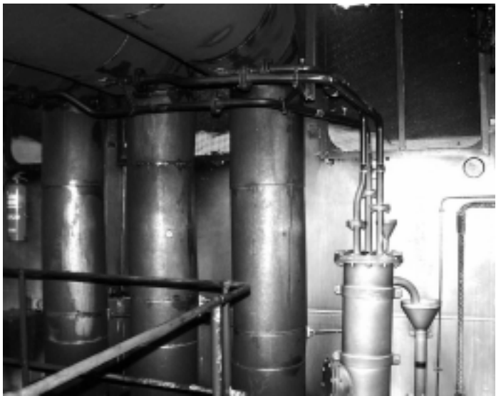
Smoke damage around diesel exhaust trunks above hydraulic room
