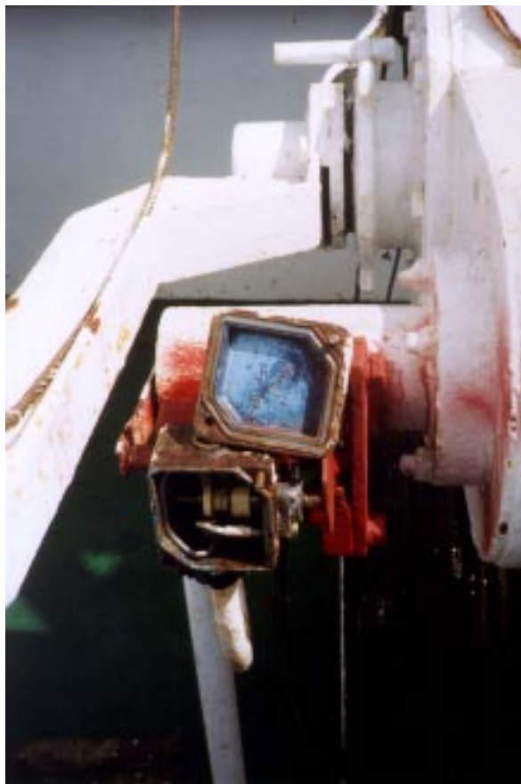
Safety cut-out switch on winch showing fractured cover plate
