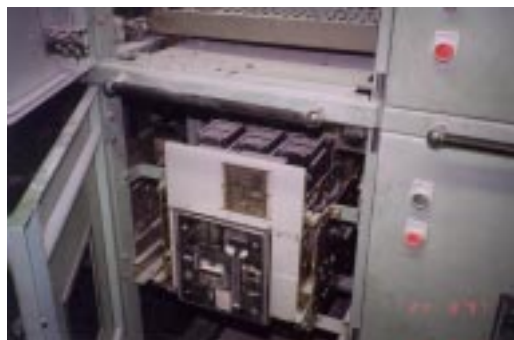
Hyundai type circuit breaker
