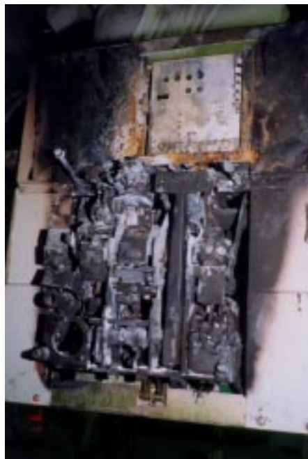
Fire Damage No.2 ACB view
