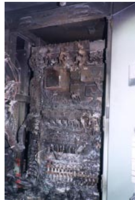
Fire damage No.2 D/G upper level
