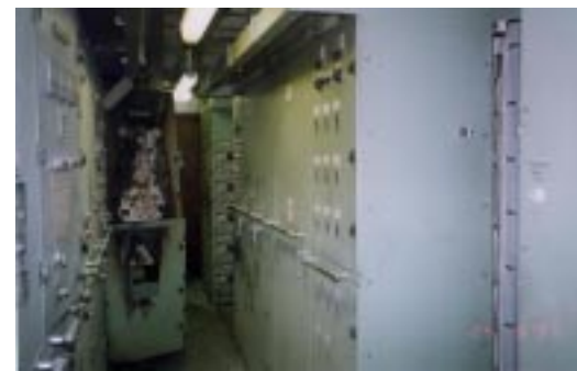
View of main switchboard room
