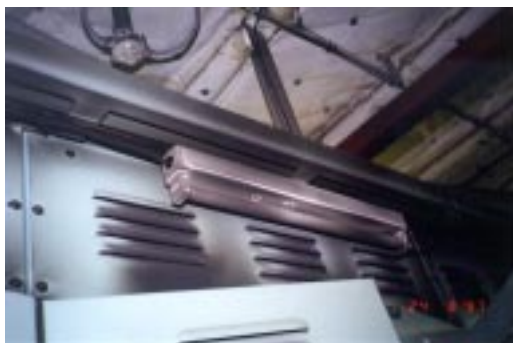
Heat detector above synchronising panel
