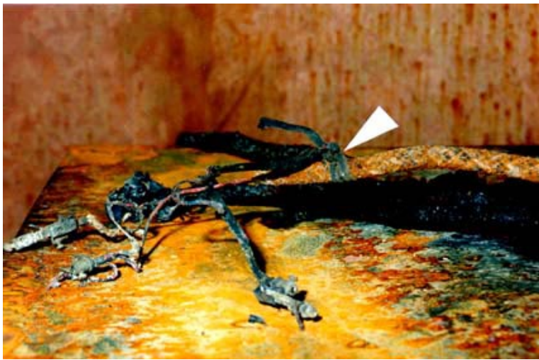
Earth strap tied with a knot to flexible conduit(arrowed)
