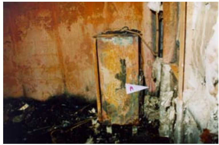
Refrigerator in corner of 1st Engineer's day room. remains of power outlet arrowed
