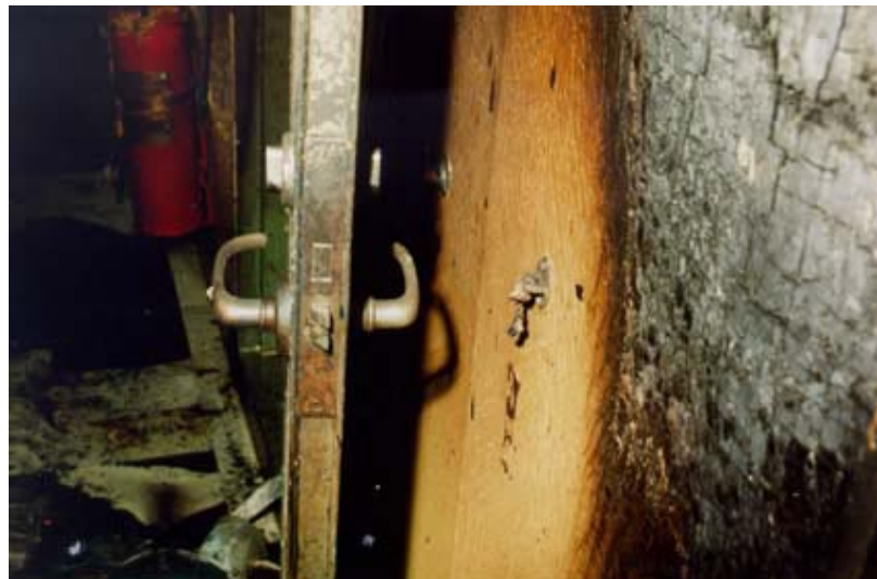
Door to stairwell at lower bridge deck showing remains of rope used to secure door in open position
