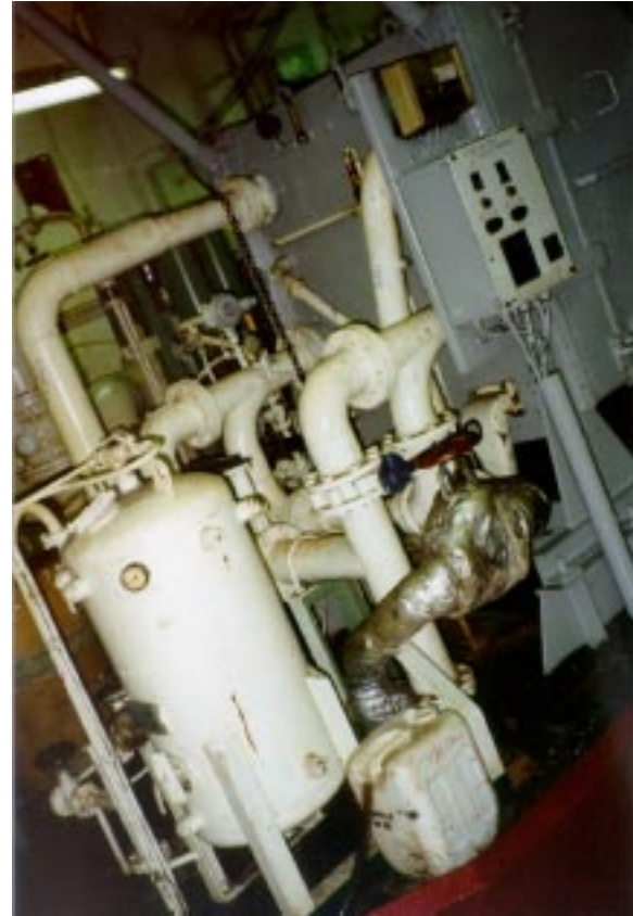
Fresh water generator
