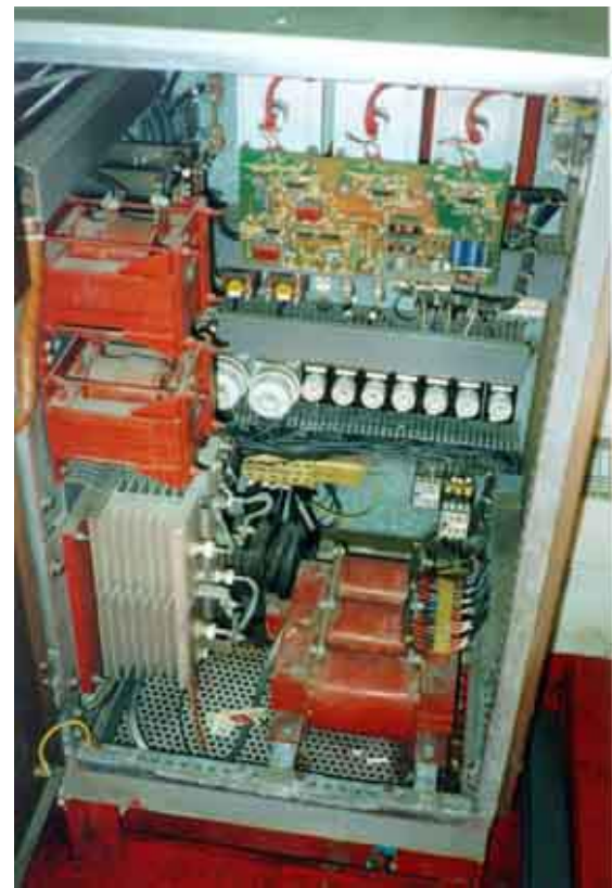
Interior of SCR60 cabinet
