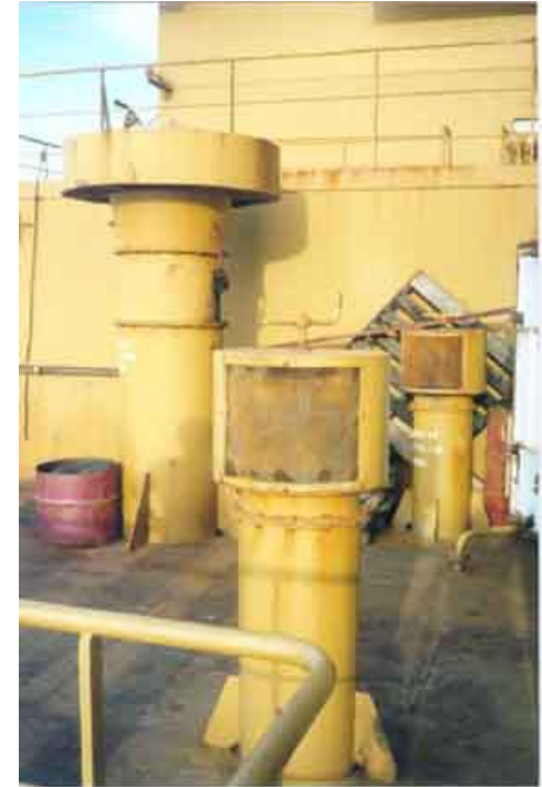
Ventilators on top of emergency generator room
