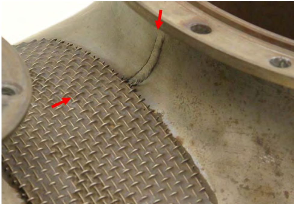
Figure A21: 'Armpit' cracking as observed in the combustion case from the Sikorsky S-76A (VH-XHS)
