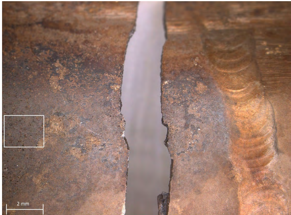
Figure A19: The internal surfaces of each 'armpit' contained similar levels of corrosion damage close to the fatigue crack origins
