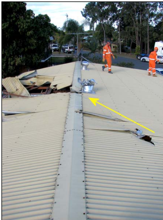
Figure 3: Damage to roof of house (arrow depicts aircraft path)
