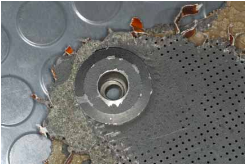
Figure 6: Typical composite panel failure around mounting point
