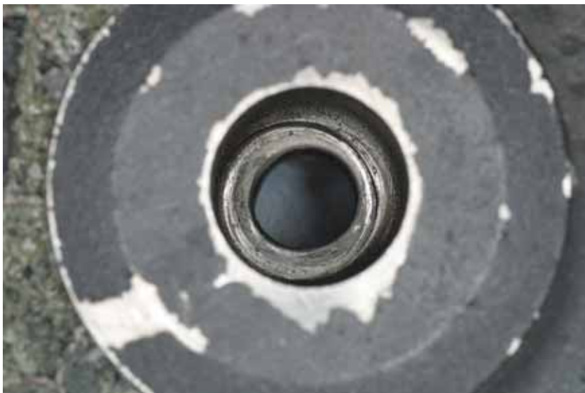
Figure 7: Elongated fastener hole showing signs of wear
