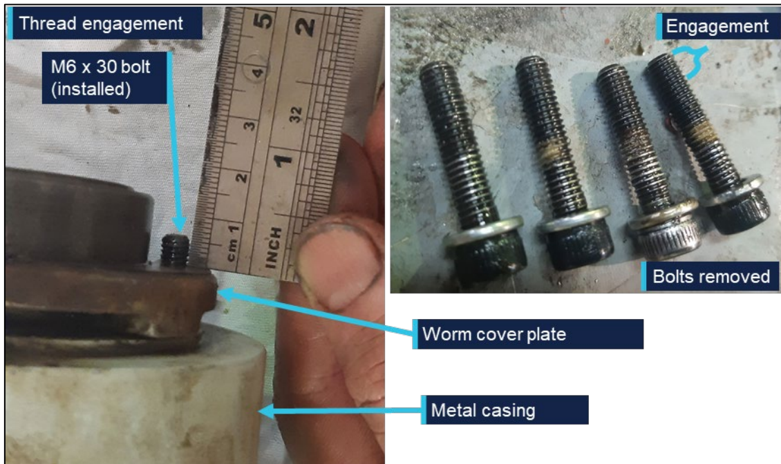
Figure 8: Securing arrangement for engine room crane traversing motor
