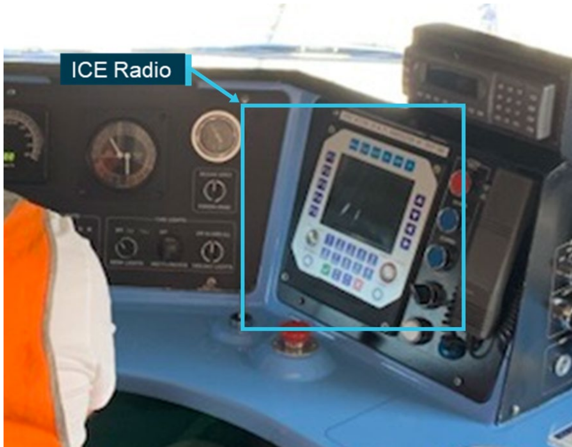
Figure 15: In cab communications equipment radio (ICE)
