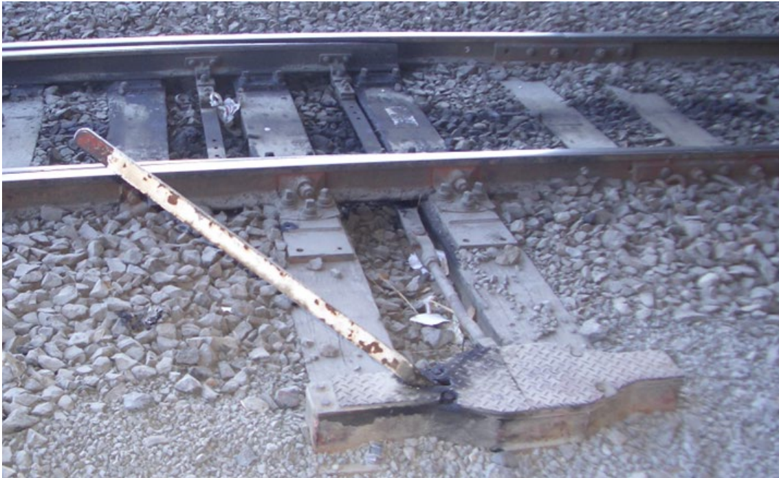
Figure 11: Example of point levers that were replaced by interlocked point motors
