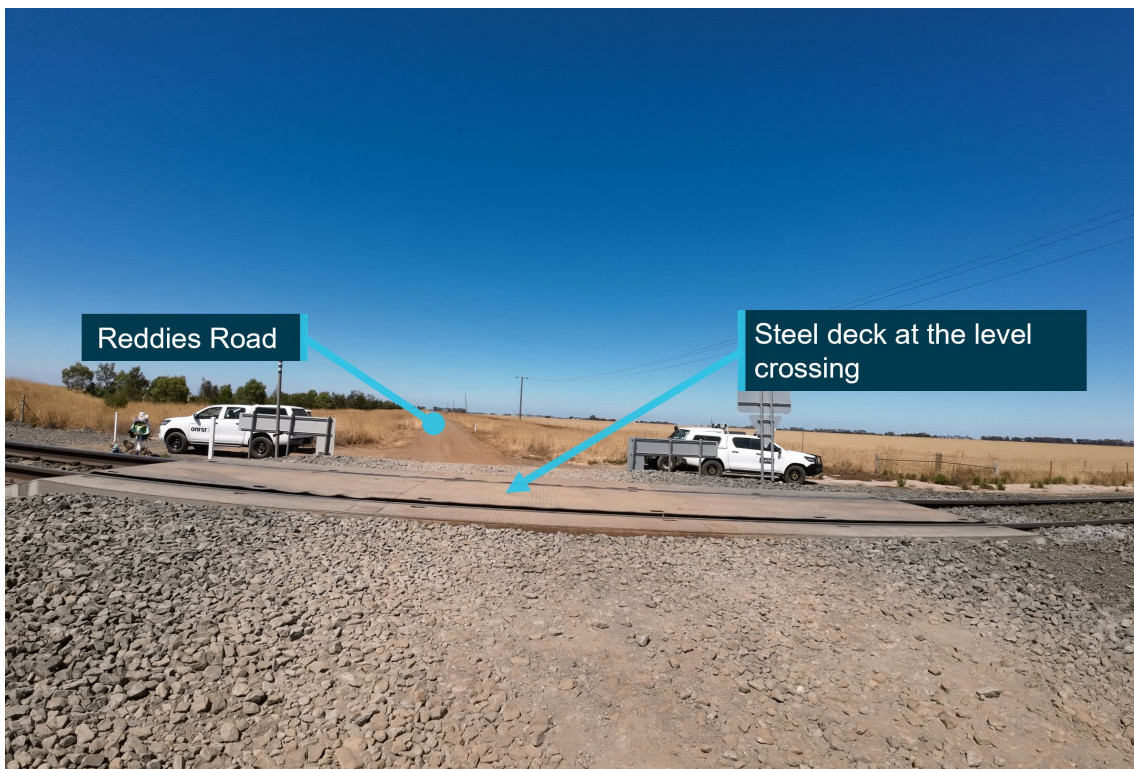
Figure 2: Steel deck installed to align the road surface with the top of the rail heads
