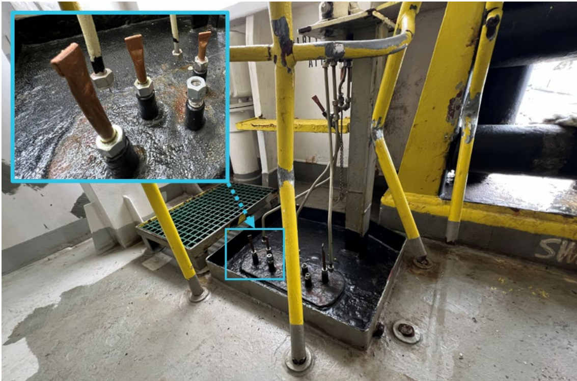
Figure 9: Viking Passama winch control emergency repair
