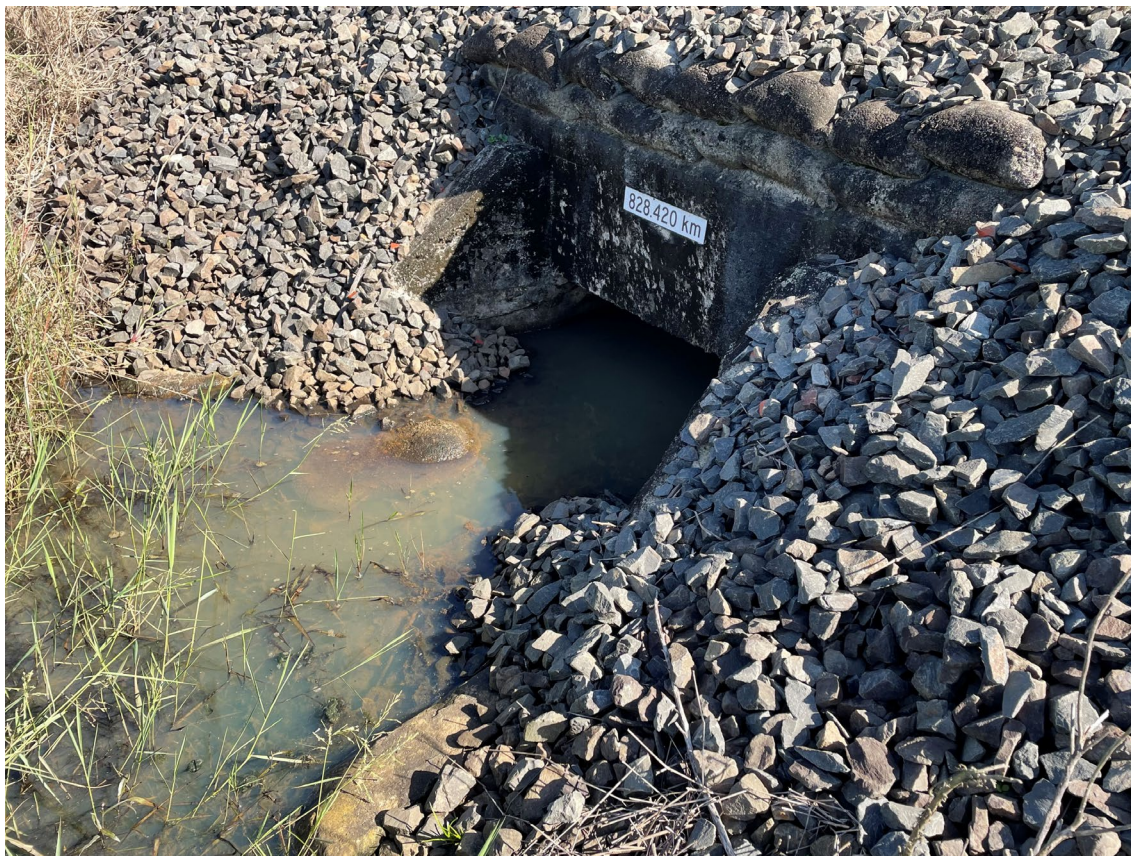
Drainage culvert directly below initial derailment site (828.420 km) showing pooled water beneath the track and formation. Source: OTSI
