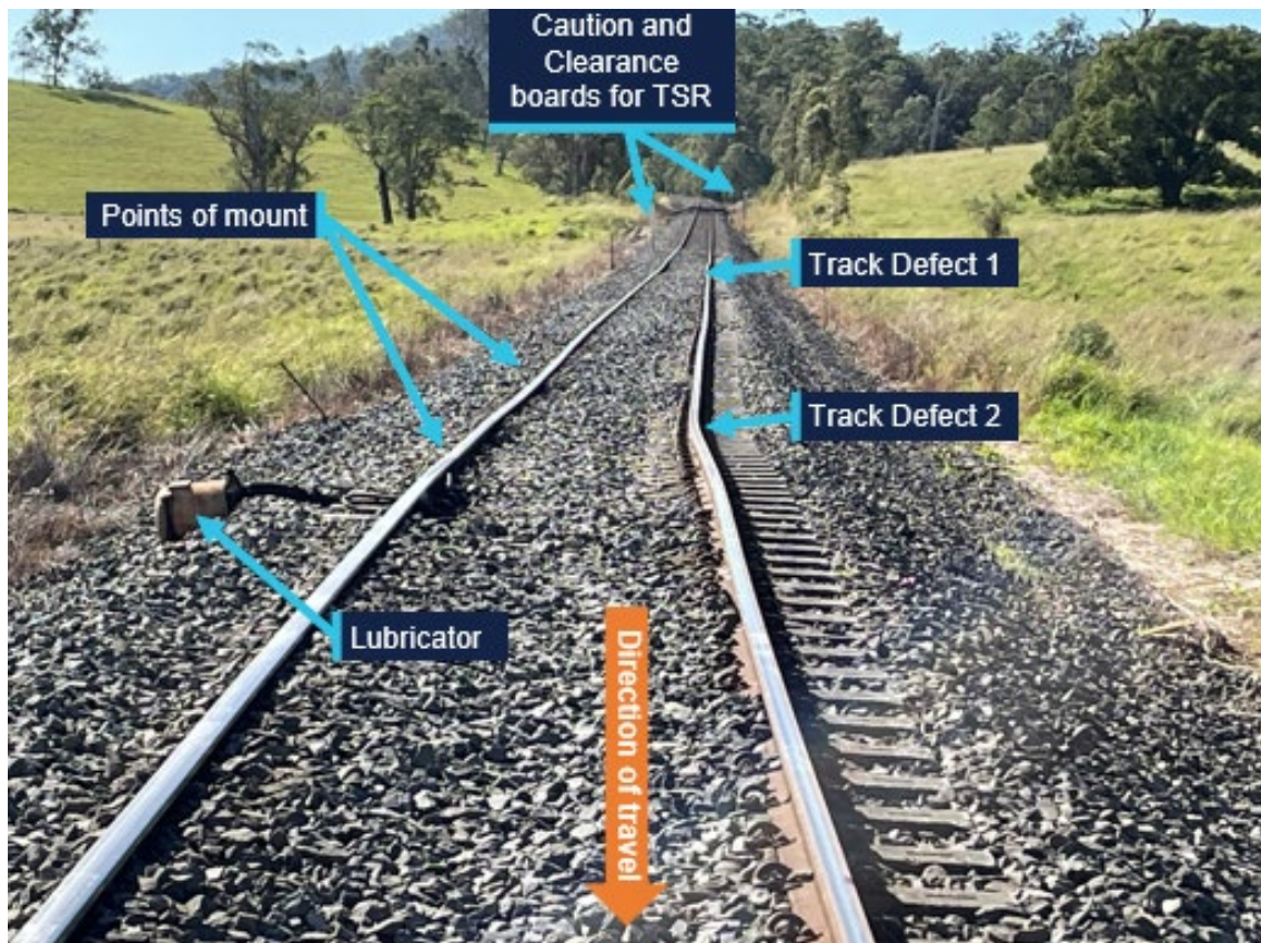
Figure 9: Post-incident view of track at point of initial derailment, facing in the down direction
