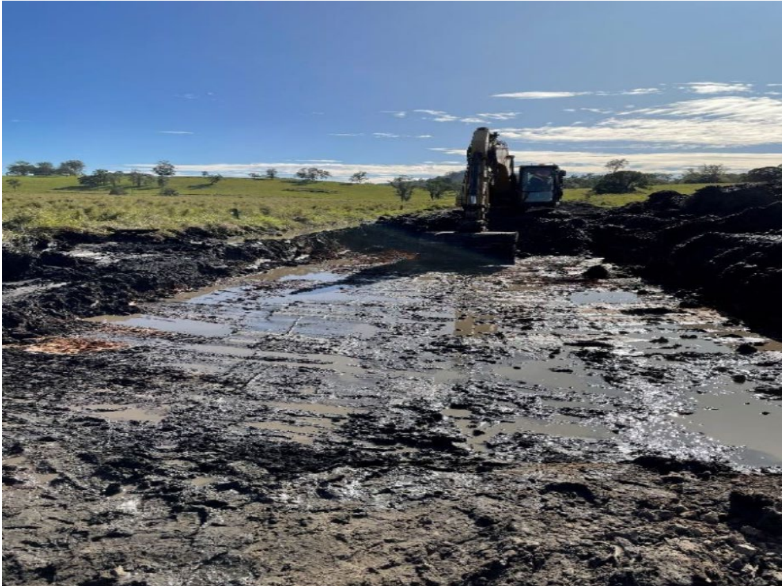
A significant amount of mud and water was found under the formation during post-derailment rectification works. Source: ARTC
