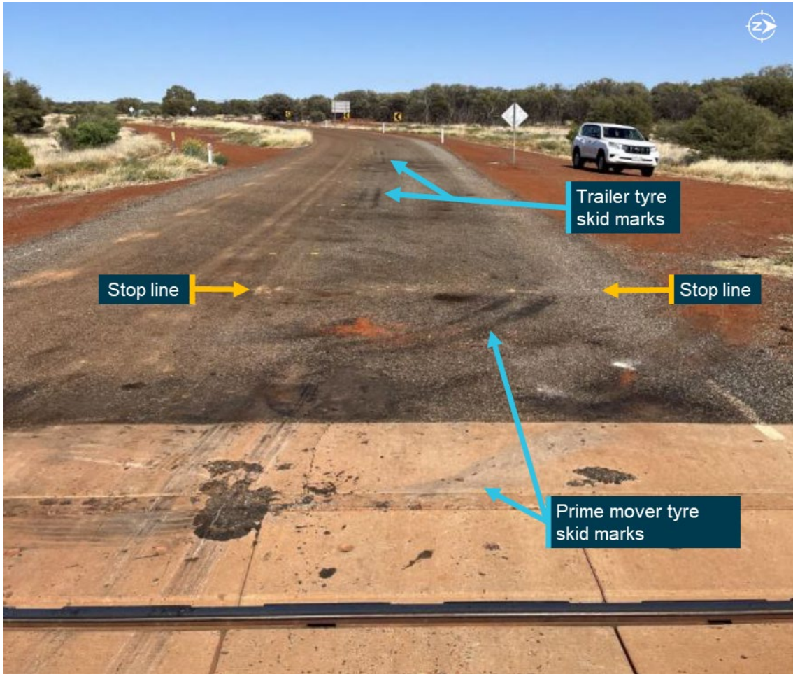
Figure 8: Faded stop line at the level crossing with skid marks evident from the emergency braking of the truck
