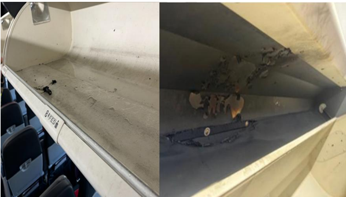
Figure 7: Overhead locker above row 7DEF where the smoke and flames were observed (left) and area behind the overhead locker showing fire damage (right)
