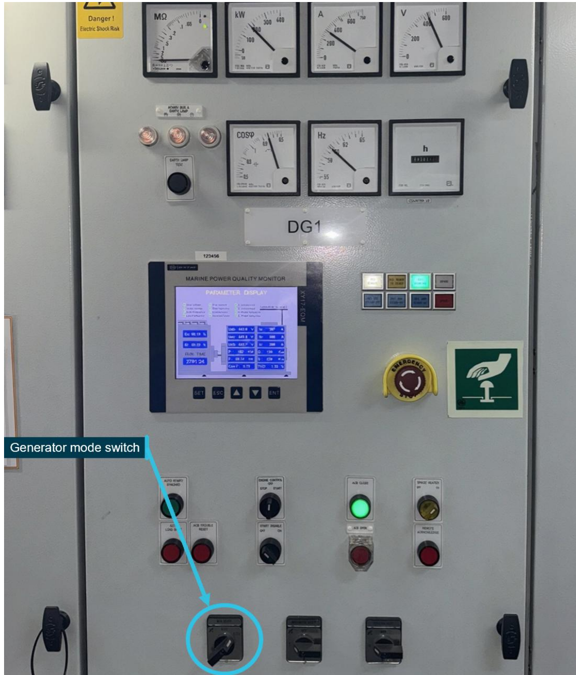
Figure 2: Control panel for diesel generator 1 (DG1)
