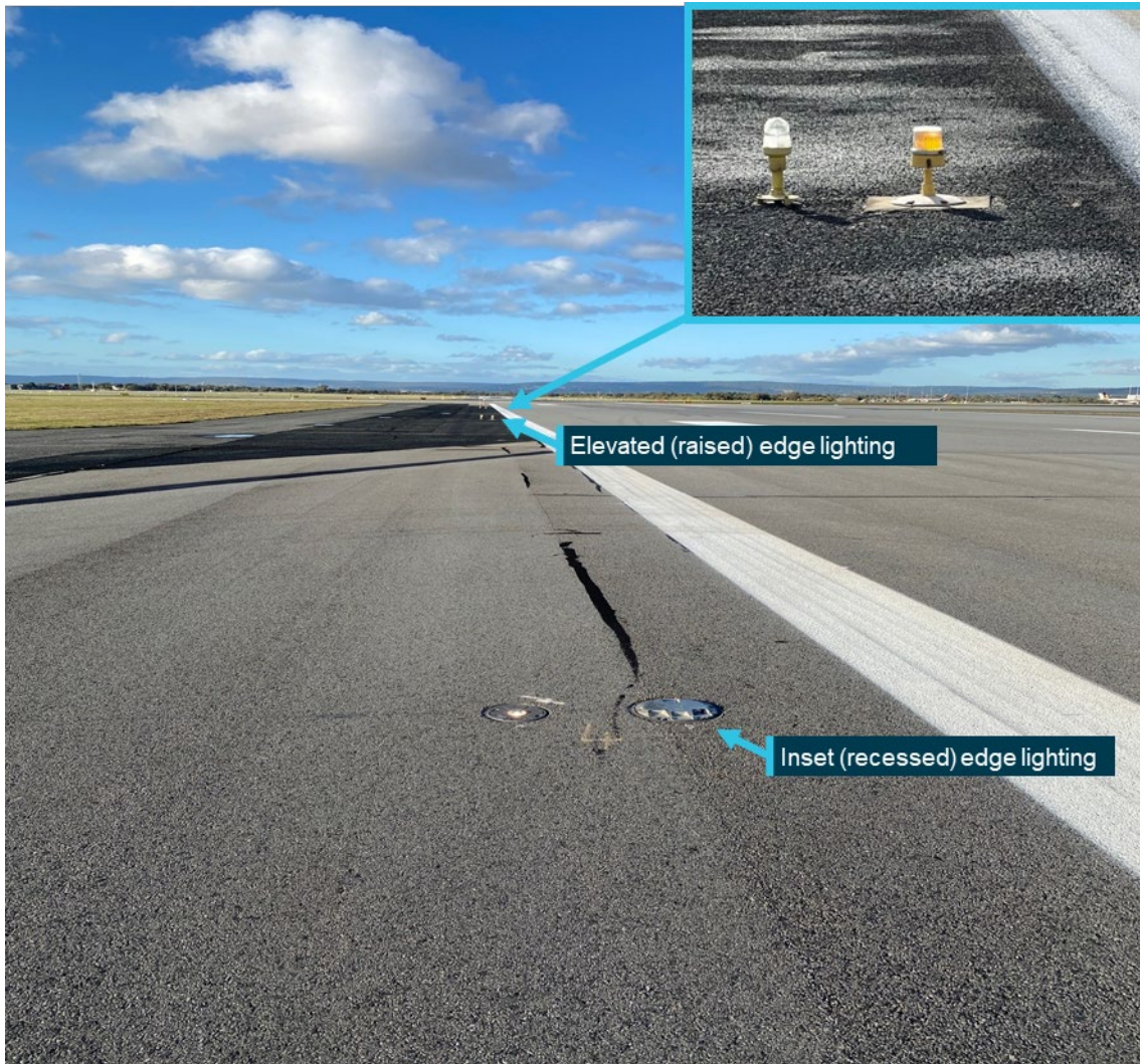
Figure 7: Runway 06 edge lighting (left side)
