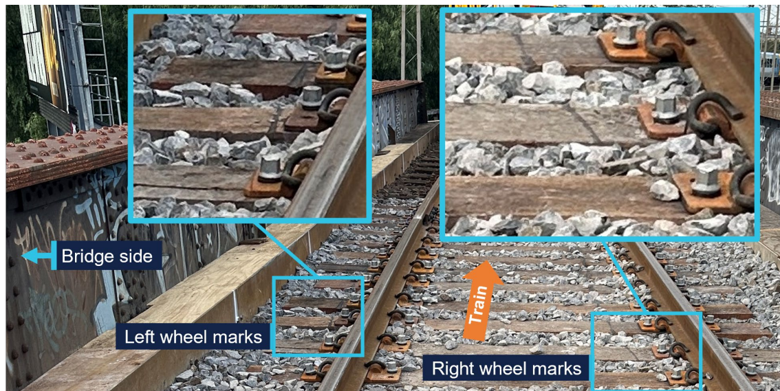
Figure 4: Marks made on sleepers by the derailed wheels
